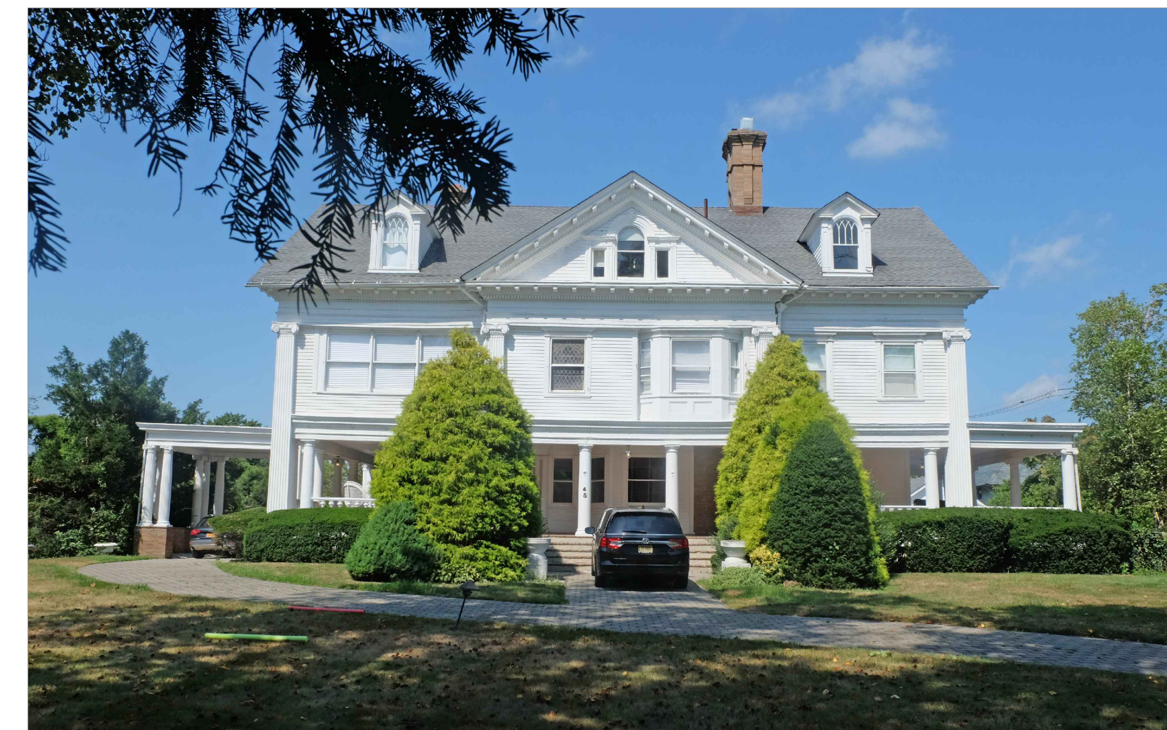
2019 CURRENT CONDITION OF HOUSE - FACADE FACING NORWOOD AVE.
